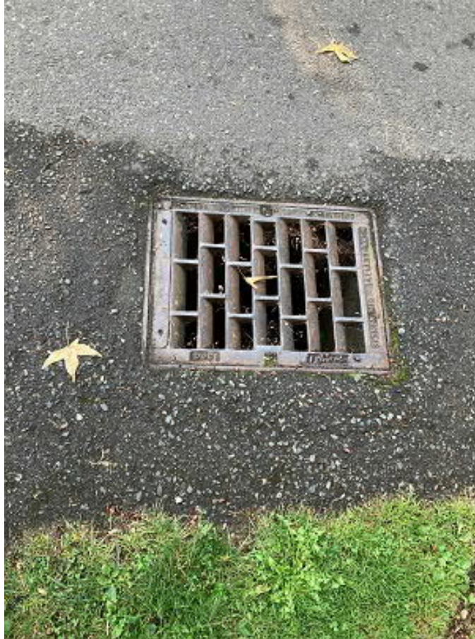
Picture 5 ROW in front of 3449 SE 36 th Street From this catch basin, water turns toward the south.
