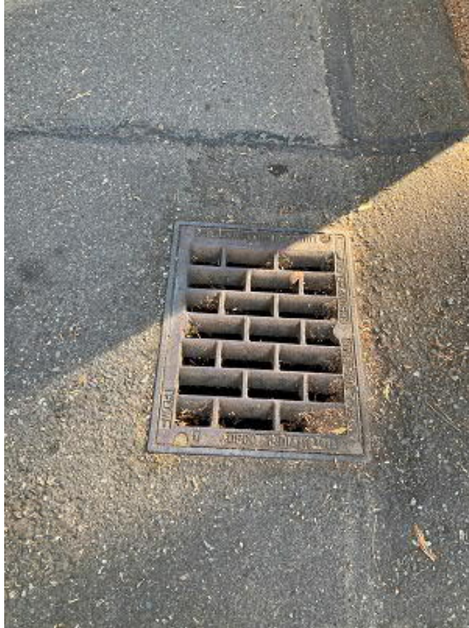
Picture 4 ROW in front of 7225 SE 36 th Street Another catch basin in line, this one under SE 36 th Street.
