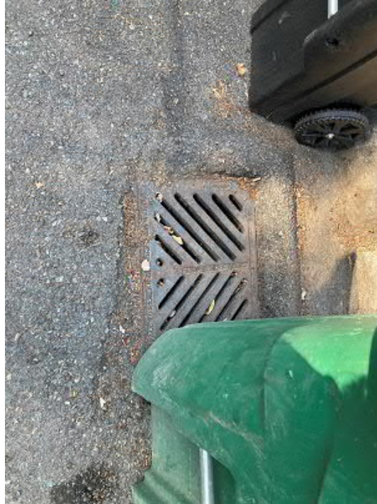
Picture 18 ROW in front of 3698 72 nd Place SE From this catch basin water heads toward the west.
