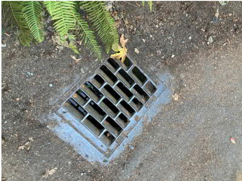
Picture 13 ROW at the NE corner of 73 rd Avenue SE and SE 38 th Street At this CB the storm drain makes a turn east under the SE 38 th Street ROW
