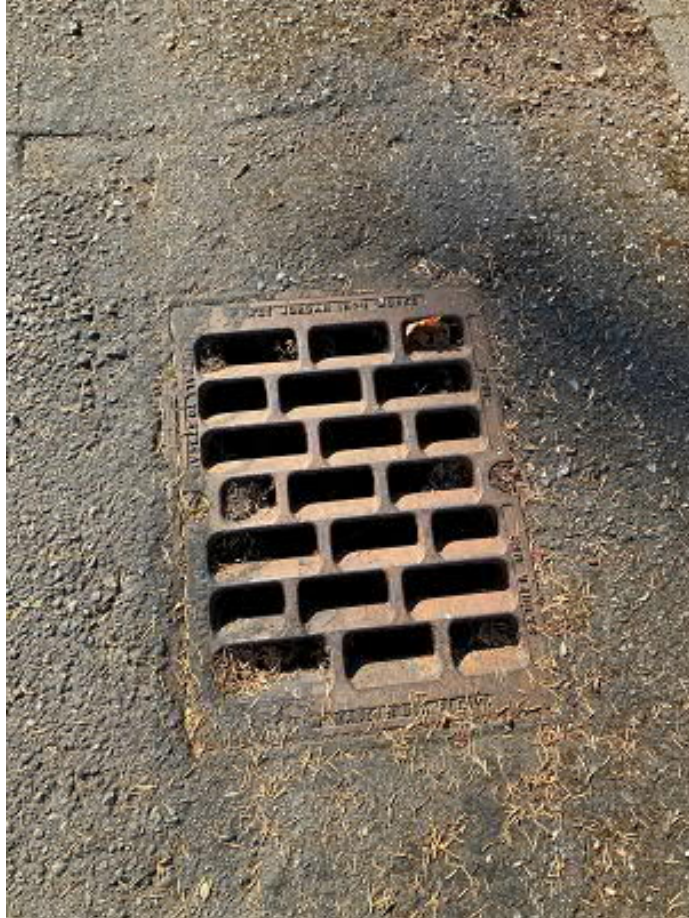
Picture 2 ROW in front of 3449 72 nd Place SE 8" DI pipe discharging toward the south leads to this catch basin.
