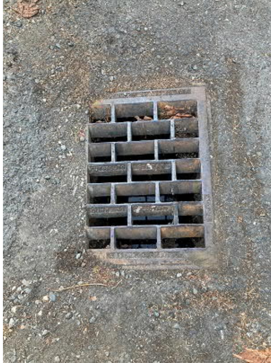
Picture 12 ROW in front of 3650 73 rd Avenue SE storm direction is due south
