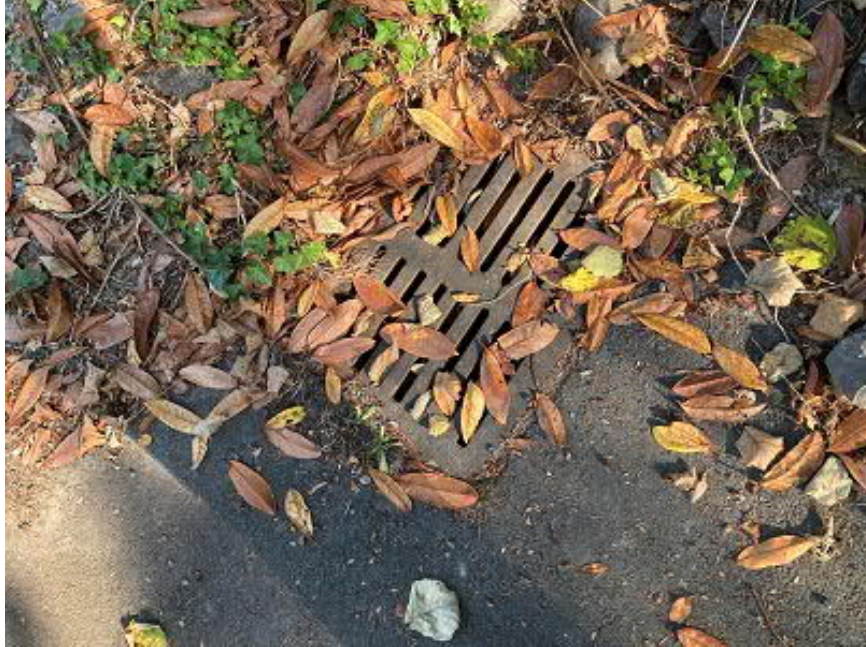
Picture 16 bottom of stairs in SE 38 th Street ROW @ 72 nd Place SE CB at the bottom of stairs. From here runoff crosses 72 nd Place SE to its west side.
