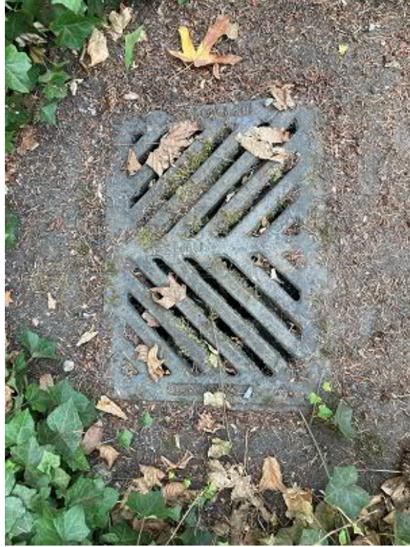
Picture 14 ROW at the sw corner of 73 rd Avenue SE and SE 38 th Street runoff heading east
